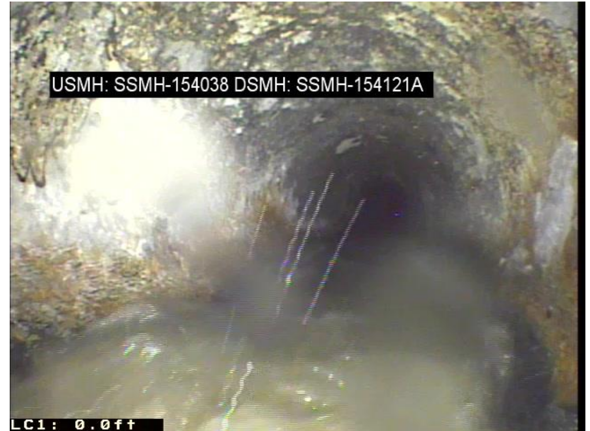
Ductile Iron Sewer Less than 20 Years Old
